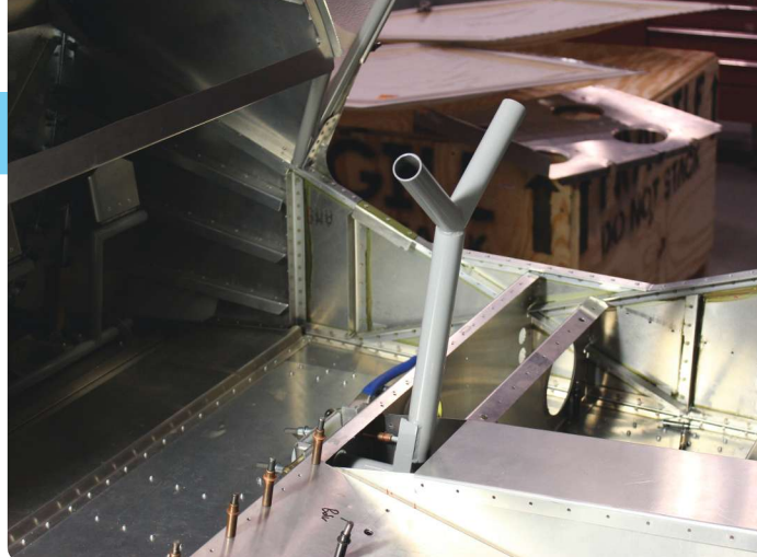
EAA staffers are currently installing the control system on the Zenith CH 750 that employees are building. We will bring you further updates on this project in an upcoming issue of Experimenter .
