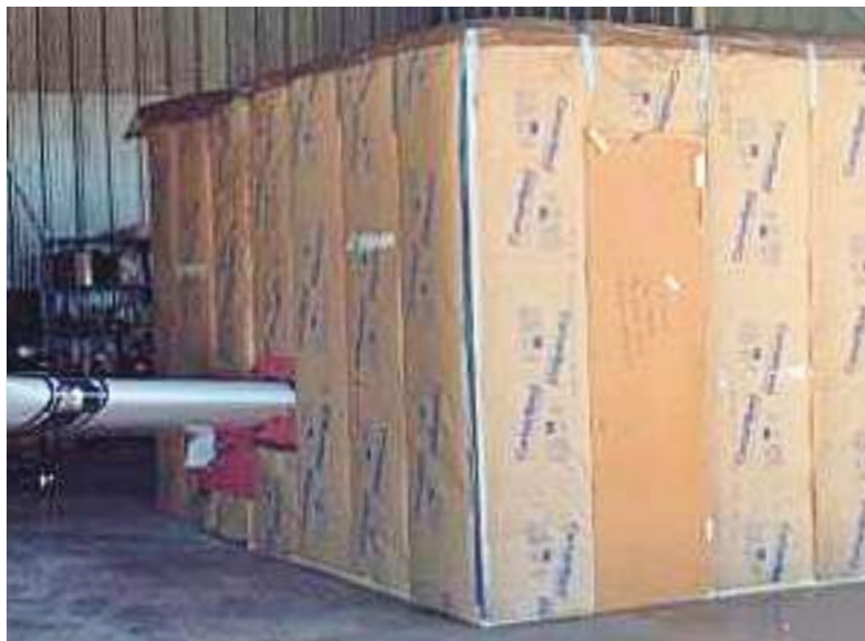
A tarp on top of the hut prevents any condensation off the metal roof from dripping on the hut.
