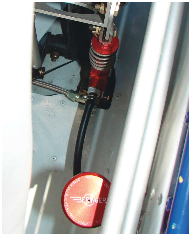
Don't neglect space for the fluid reservoir and lines. Plan ahead for every component, as in this Air Cam.
