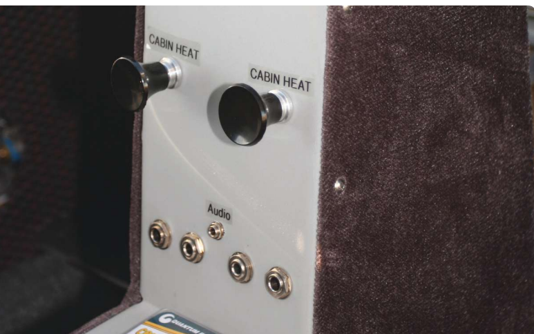
The console mounts pilot/co-pilot heater controls.
